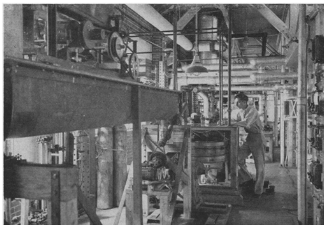
FIG. 3. Slurry mixer and its feeder at left, 3-in. slurry feed conveyor and drive in lower left center, and 3-ft. diameter rotary vacuum horizontal filter at right.
